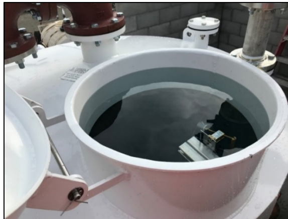
New potable water tank installed Piping Renovation – Phase 9
