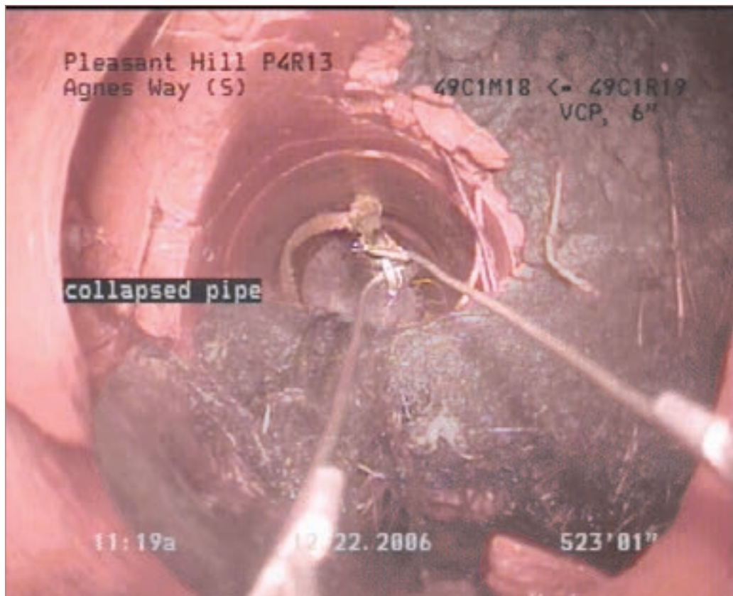
TV inspection of the collection system helps to guide sewer renovation plans.
