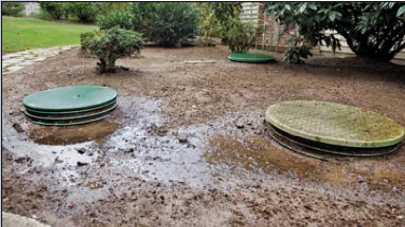
A septic tank overflow
