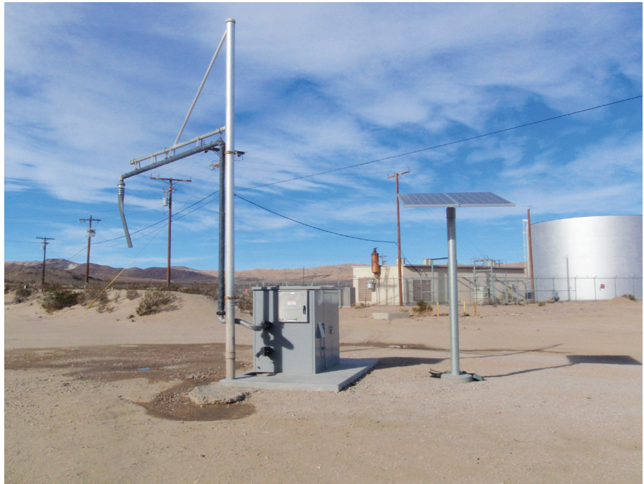
An Automated Recycled Water Fill Station like this one will be operational by June 2016.
